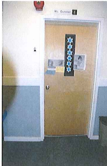
Middle School: Door Hardware is not ADA Accessible
