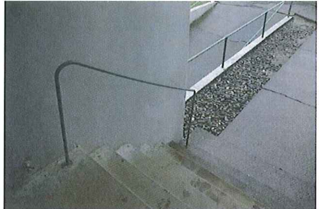
Middle School: Handrail is not Code Compliant
