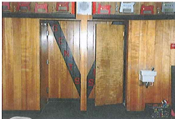
Gymnasium: Restroom Doors are not ADA Accessible
