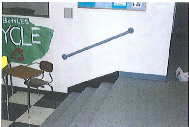
High School: Handrail Extension Does not Meet Current Standards
