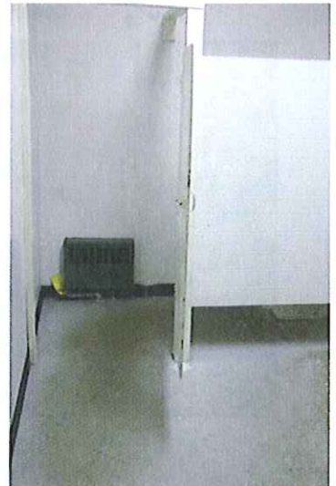
Gymnasium: Toilet Stall is Not ADA Accessible
