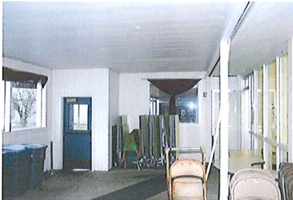
Multipurpose Building: Foyer Needs Egress Lighting
