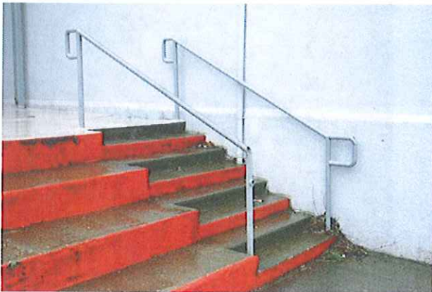
Middle School: Handrail Extensions do not Meet Current Standards
