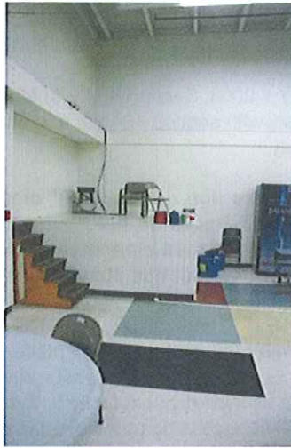
Multipurpose Building: Platform needs a guardrail
