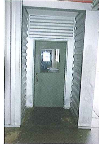
Multipurpose Building: Entrance is not ADA Accessible
