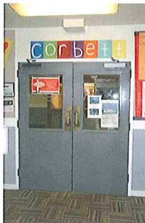
Middle School: Doors Pulls are not at ADA Accessible Height
