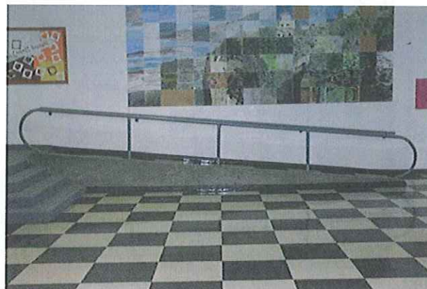
High School: Ramp Slope Exceeds ADA Standards
