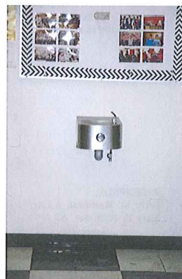
High School: Drinking Fountain is not ADA Accessible
