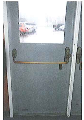
Gymnasium: Panic Hardware Does not Meet Current Day Standards
