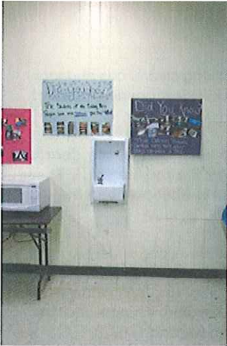
Multipurpose Building: Drinking Fountain is not ADA Accessible
