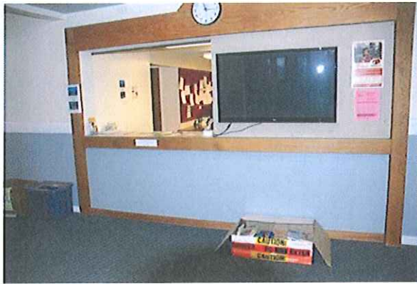
Middle School: Counter Height is not ADA Accessible
