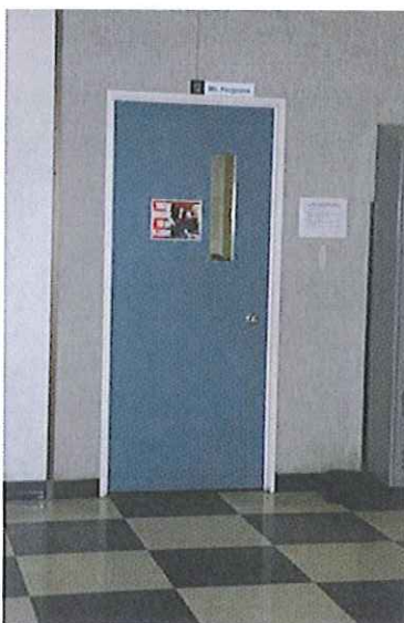
High School: Door Hardware is not ADA Accessible
